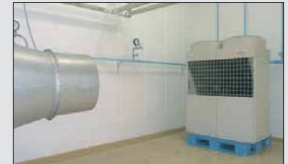
Shower Test Room
