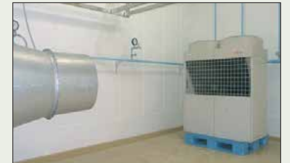
Shower Test Room
