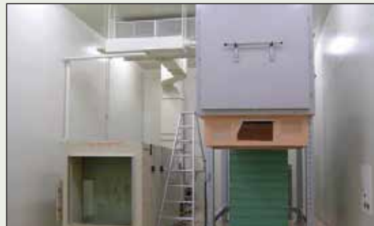
Air Volume Measurement Room
