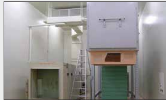
Air Volume Measurement Room
