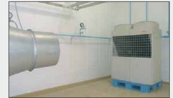
Shower Test Room
